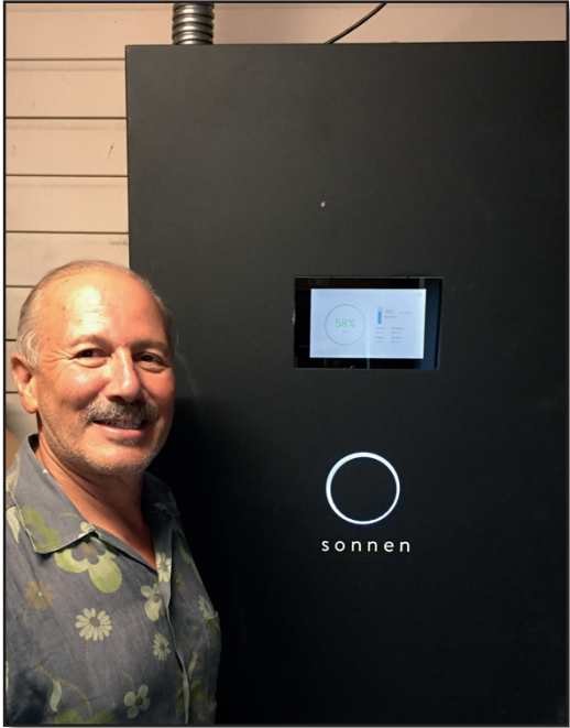
The 10 kWh sonnen ecoLinX smart energy management system installed in the cyberManor garage next to the circuit panel and PV Inverter.
