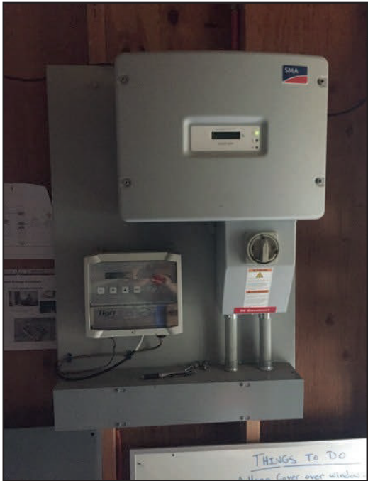
SMA America PV Power Inverter with the TiGo Solar Energy Monitoring.
