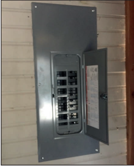
Main circuit breaker panel for all the town house loads.
