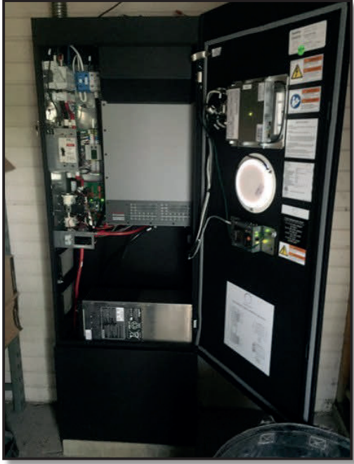
Inside the 10 kWh sonnen ecoLinX smart energy management system – the five (5) x 2 kWh batteries are located in the bottom of this enclosure.
