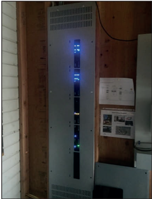
Control4 centralized lighting panel for the showroom.
